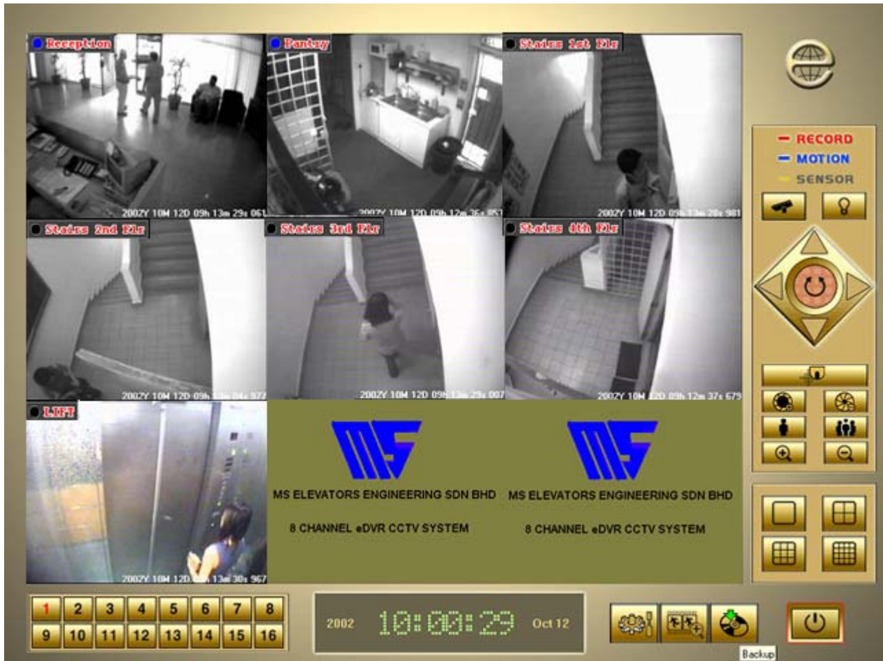
Typical Monitor Screen for CCTVs
